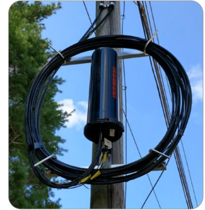
Coil Bracket holds excess ADSS cable
