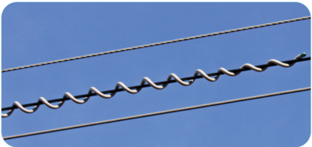
Spiral Vibration Damper on ADSS Cable
