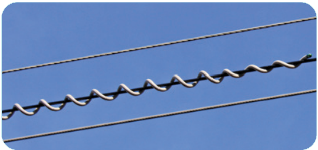
Spiral Vibration Damper on ADSS Cable
