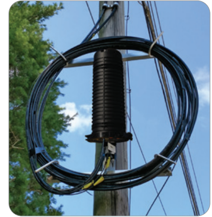
Coil Bracket holds excess ADSS cable
