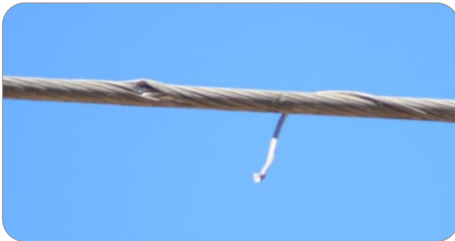
Figure 1—Damaged conductor stranding
