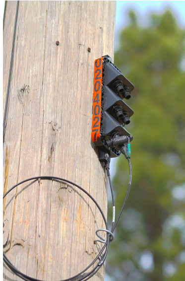
Figure 5—Multiport terminal with hardened drop connectors installed.
