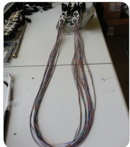
Photograph 6—Mid-Cable Access Arrangement Sealed Closure of a 576F WTC Fiber Cable
