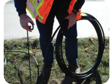
Photograph 21—WTC 432F PSP Cable Storage Coil
