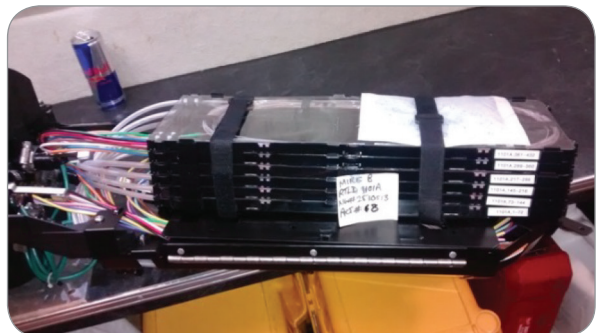
Photograph 5—Network Splice Trays 432F WTC and 144F Loose Tube Cables
