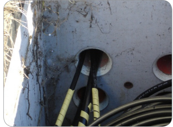
Photograph 3—Underground Duct with Two 432F and One 864F WTC Cables
