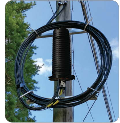
Coil Bracket holds excess ADSS cable
