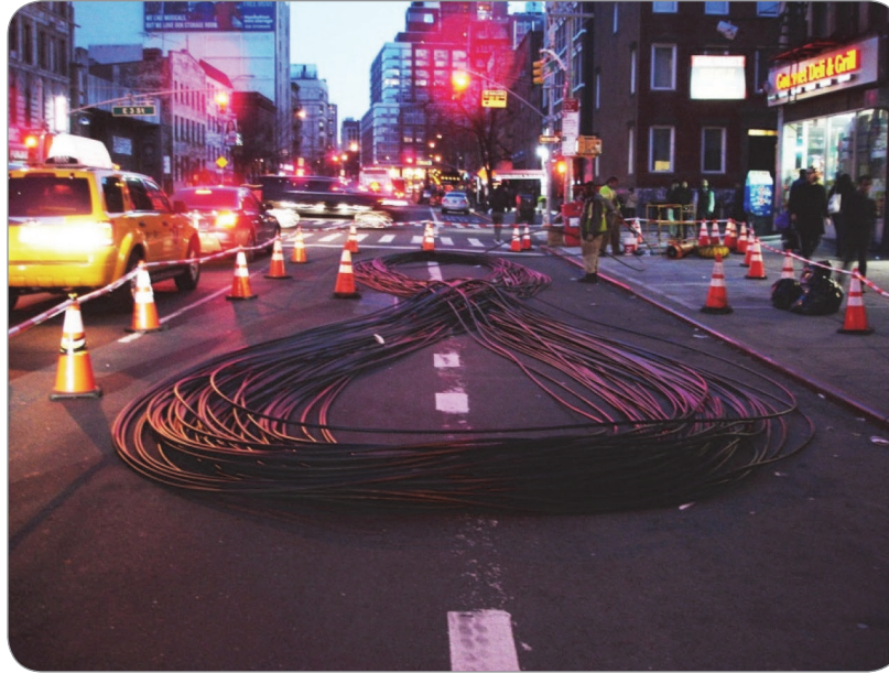
7,000 feet of 1,728F WTC in Figure-8 Coil
