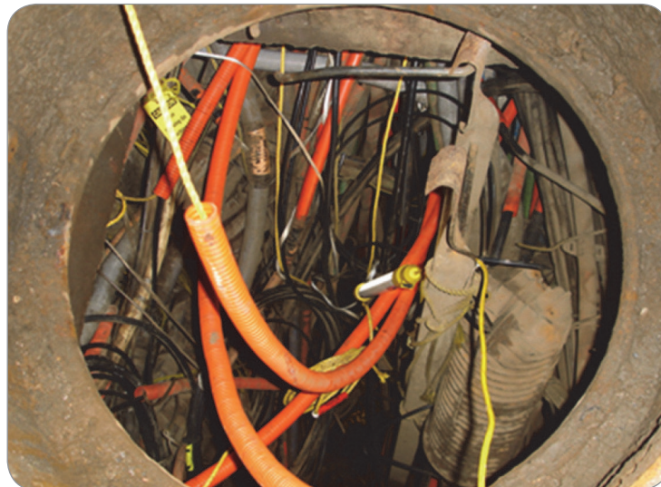
Congested NYC Manhole with 2-inch Innerduct Pathway
