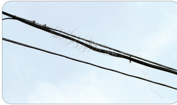
Figure 3: Loosening of lashing wire
