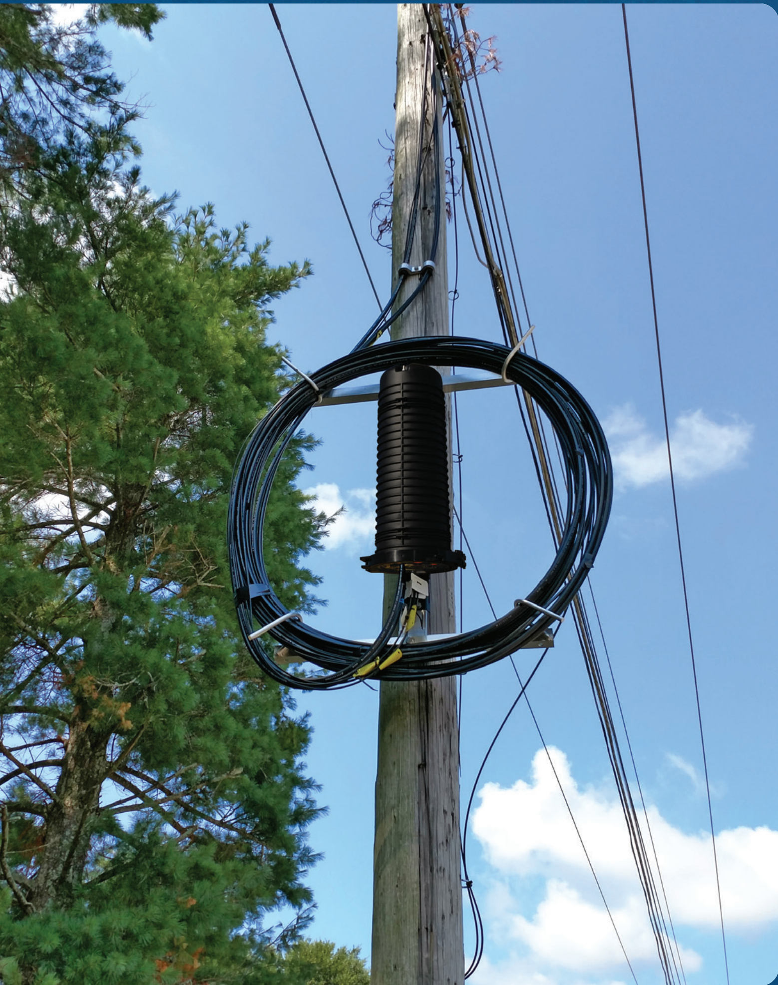
TRANSITION INTO SUBSTATION
