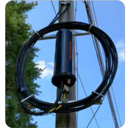
Coil Bracket holds excess ADSS cable
