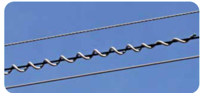
Spiral Vibration Damper on ADSS Cable
