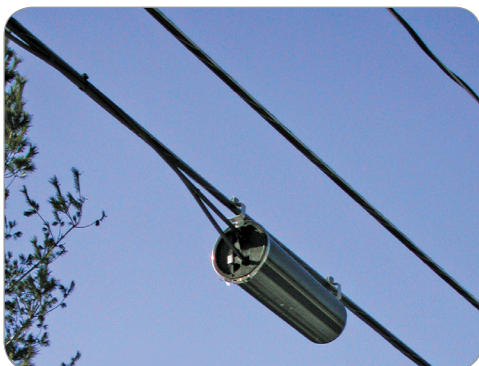
Sealed Splice Closure
